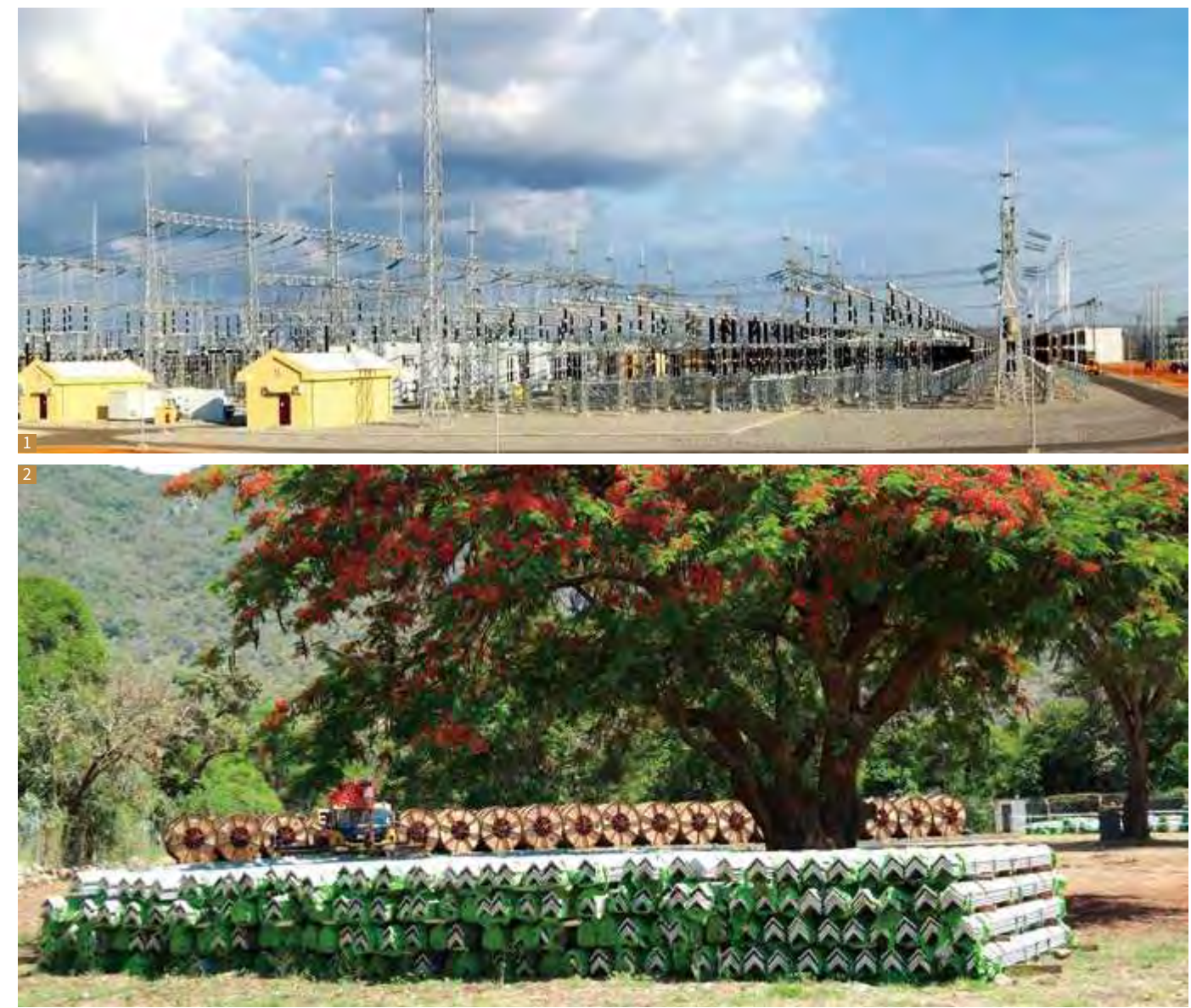
1 The Largest Power Transmission Project in Angola so far – Angola SK 400kV Transmission Line
