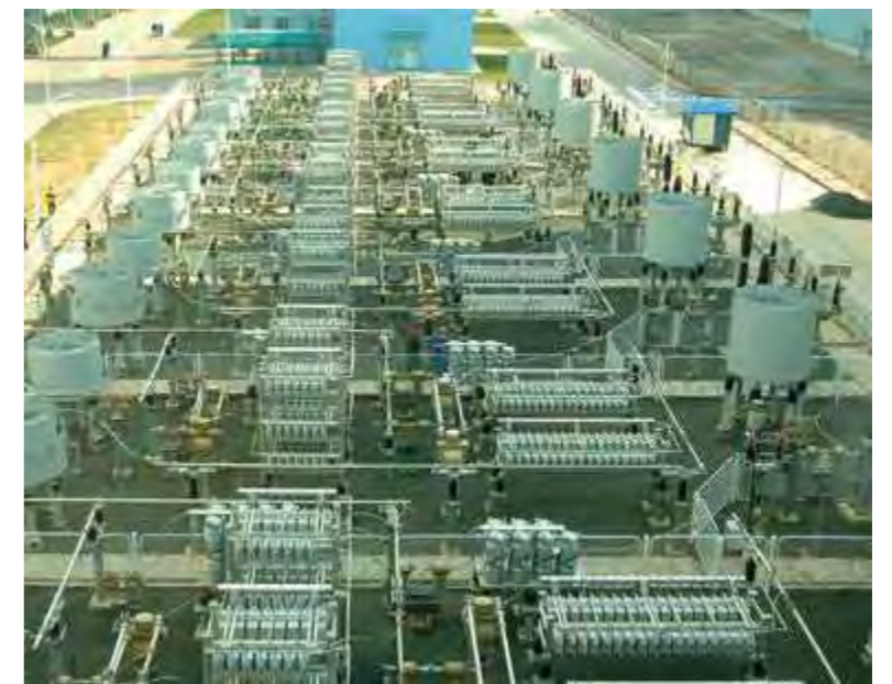
Panorama of Blocking Filters at Datang Tuoketuo Power Station
