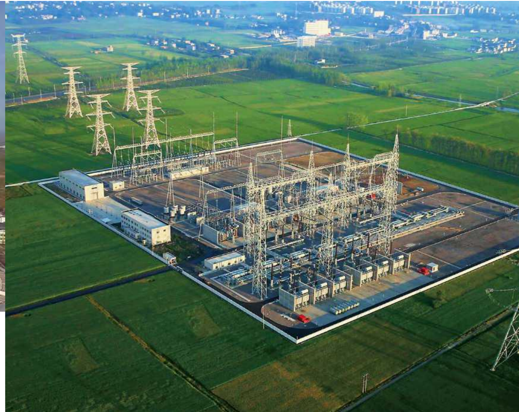
Huainan 1000KV Substation - Huainan to Shanghai UHV AC Transmission Line and Substation Project of "Anhui to East China Power Transmission Program"
