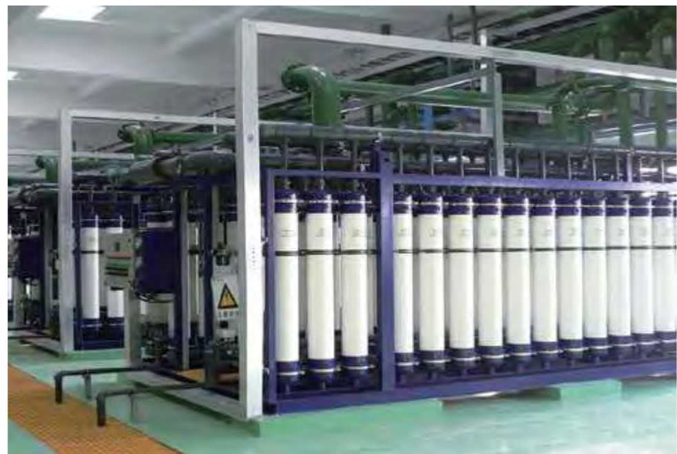
Seawater Desalination System of Hebei Wangtan Power Plant
