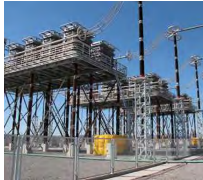
The World's First 1000kV Compensating Device put into operation in Jindongnan Substation
