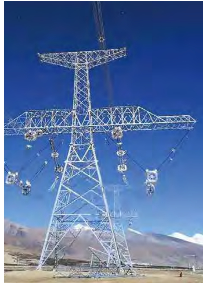
Tibet's High-altitude UHV DC Test Base Project
